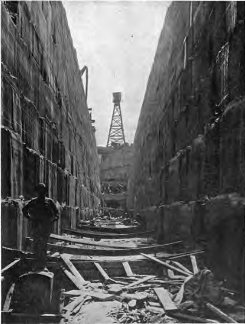
PLATE 52.—View of Trench Channeled in Bluestone and Shale for Pressure Aqueducts, just before Placing Concrete. Cableway Used for Removing Excavation, etc.
